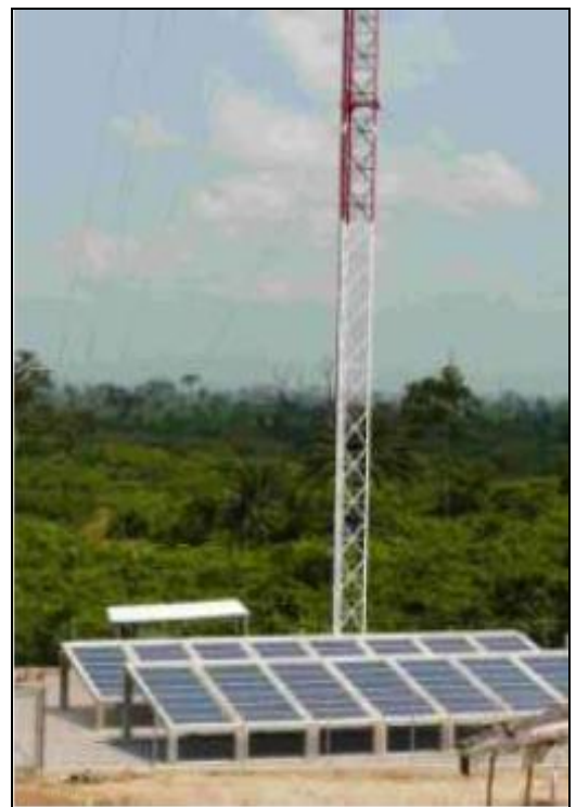
Figure 2: Solar powered BTS – Côte d'Ivoire
