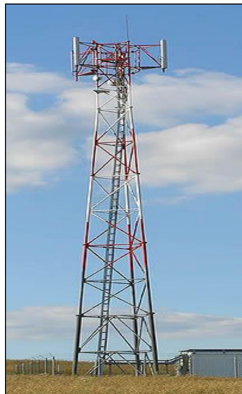
Figure 1: Standard Mobile Base Station
